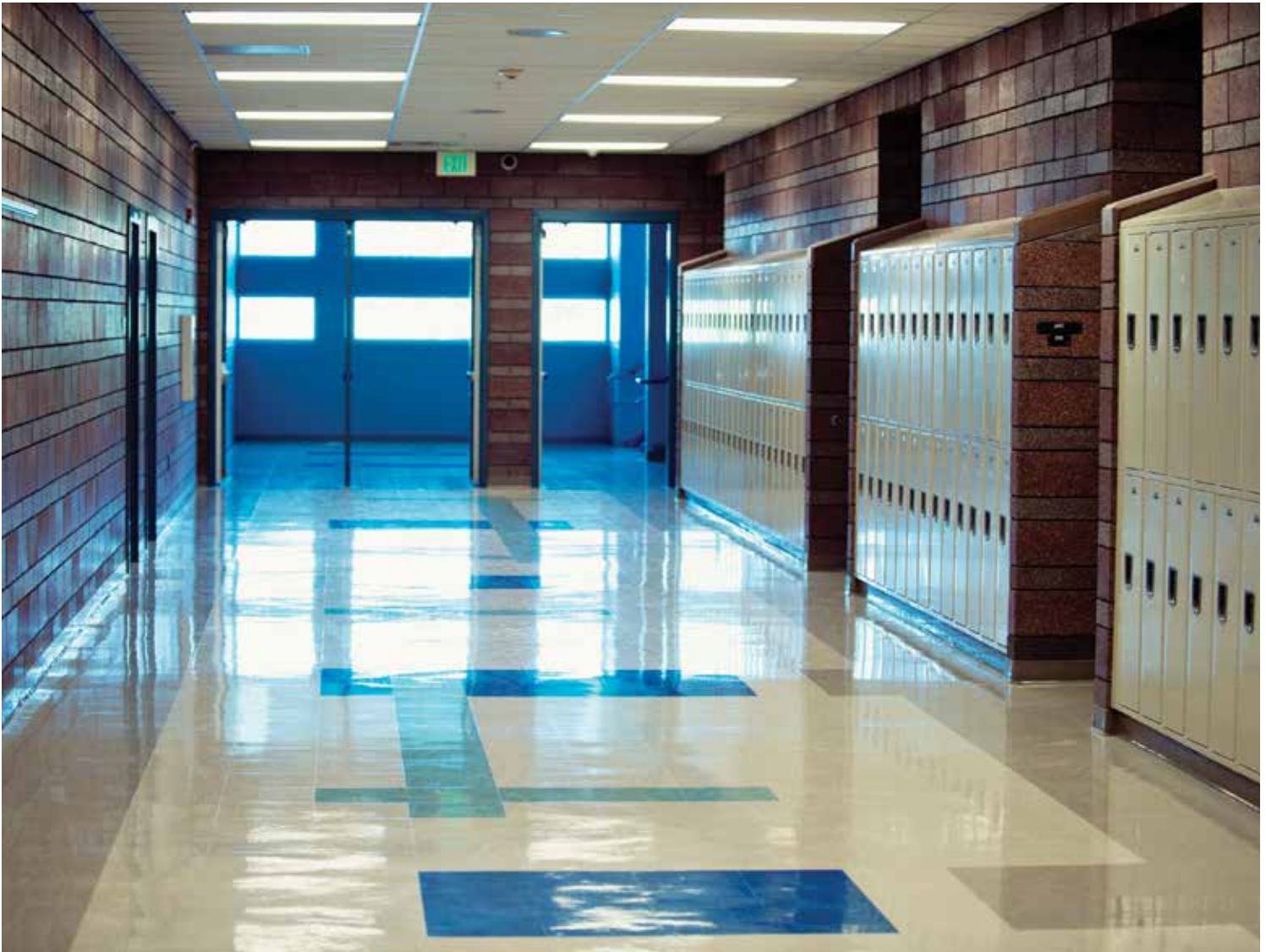
Atlas Enclosures for IP Speakers Are an Integral Part of a ControKom® 2.0 Messaging System Deployed in a School
