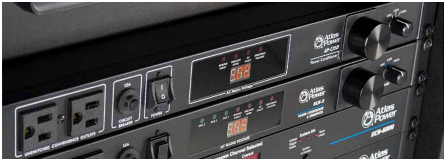
Atlas Power Solutions Are Easily Integrated Into Any Standard Equipment Rack
